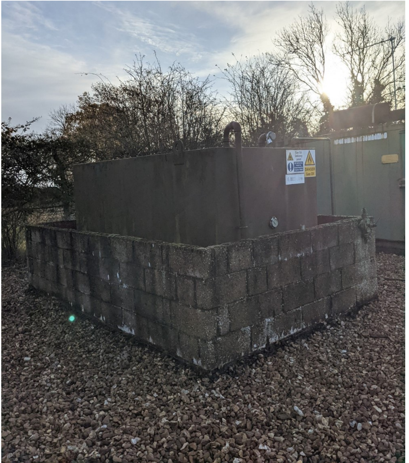
Photo 1: Waterbeach WRC fuel tank
